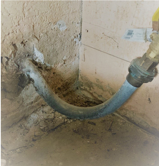
Photo of a lead service line in a home in North Platte, NE.
